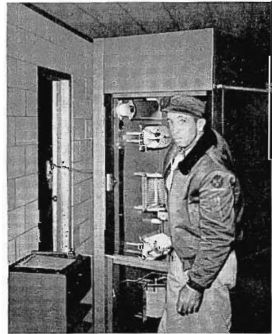
FIG. 7. Tom McFerrin, chief engineer for WCBI and The Mid-South Network, inspects the phasing gear before sliding phasing cabinet into position beside the BTA-1M 1 kilowatt transmitter at the WCBI transmitter.
