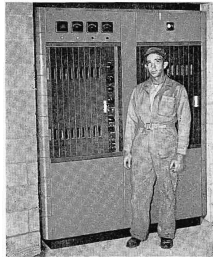
FIG. 6. Shown in front of the BTA-1M and the phasing cabinet, is Tom McFerrin, chief engineer of WCBI, who supervised the complete installation of the new kilowatt plant. The two cabinets will be framed with moulding around the edge of the opening to form a perfect installation from standpoint of convenience and appearance.
