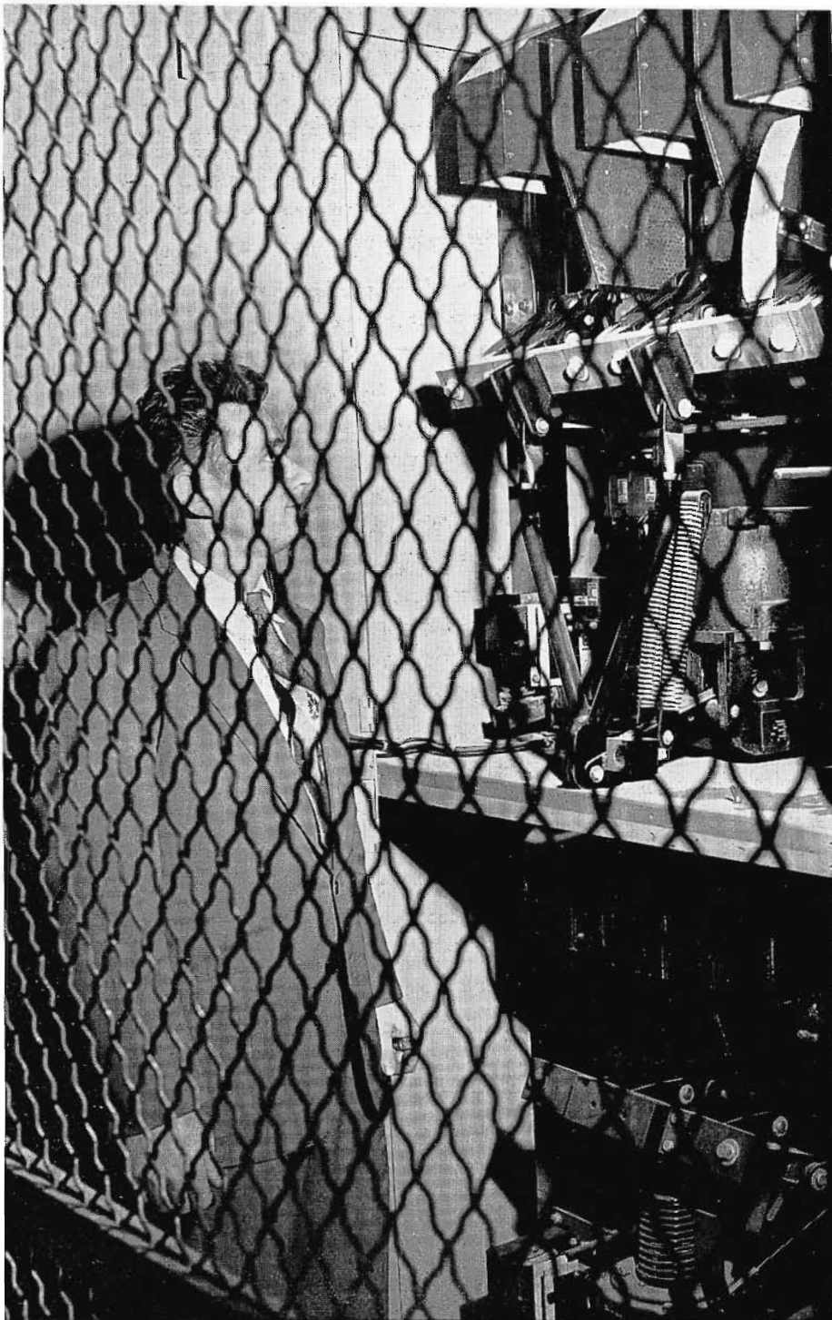
FIG. 8. Jay Cleaves, Building Chief Engineer, shows 3000 amp. and 2000 amp. main electrical breakers with fronts removed.
