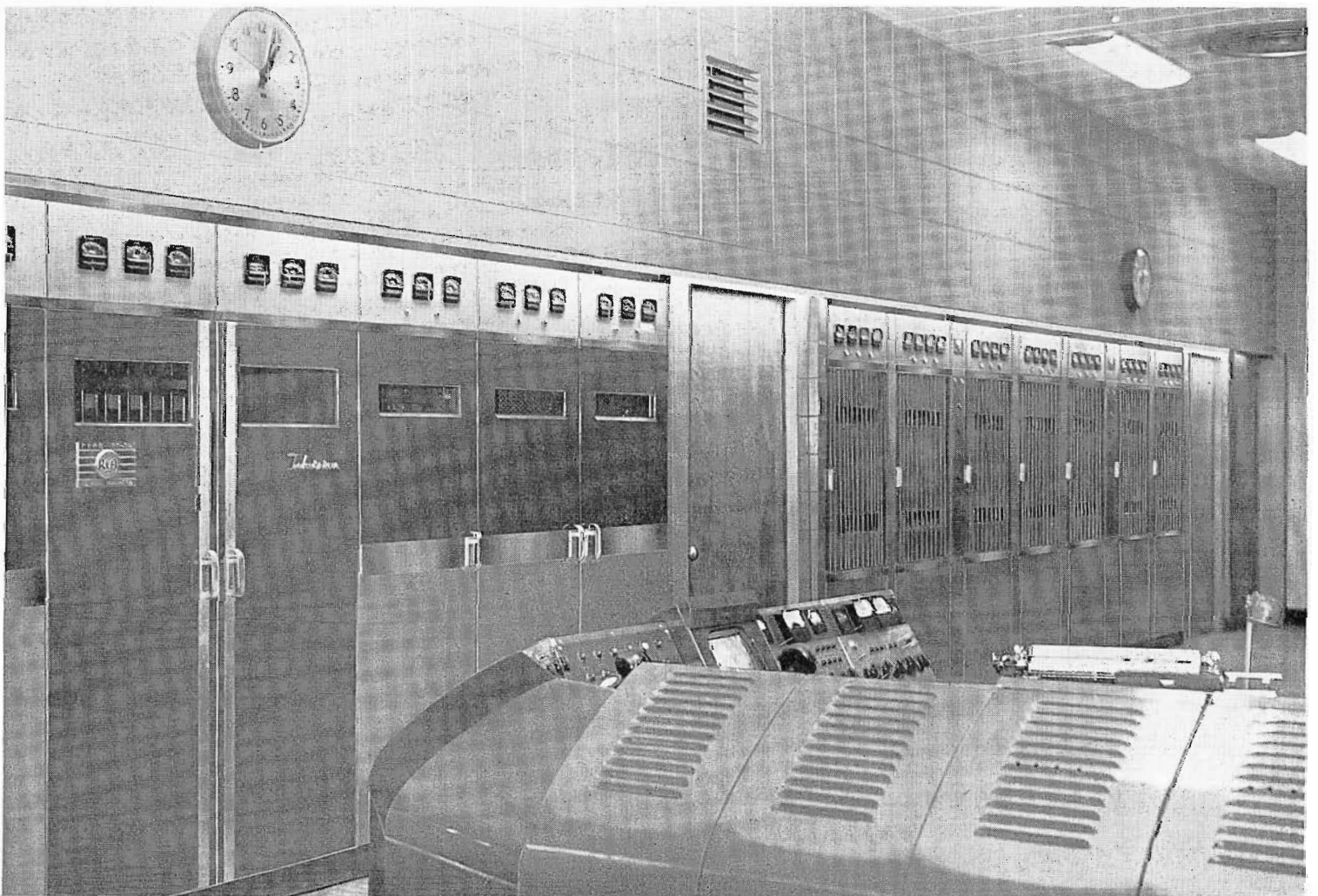
FIG. 29. TT-5A standby transmitter on the left and high power TT-50AH on the right are both monitored by one control console. TV master control extends to the lower right.
