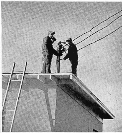
FIG. 1 (left). Power crews connect power to the WCBI transmitter building preparatory to installation of the "all RCA" installation of radio and TV for WCBI. The new site is four miles northeast of center of Columbus, on Highway 12.
