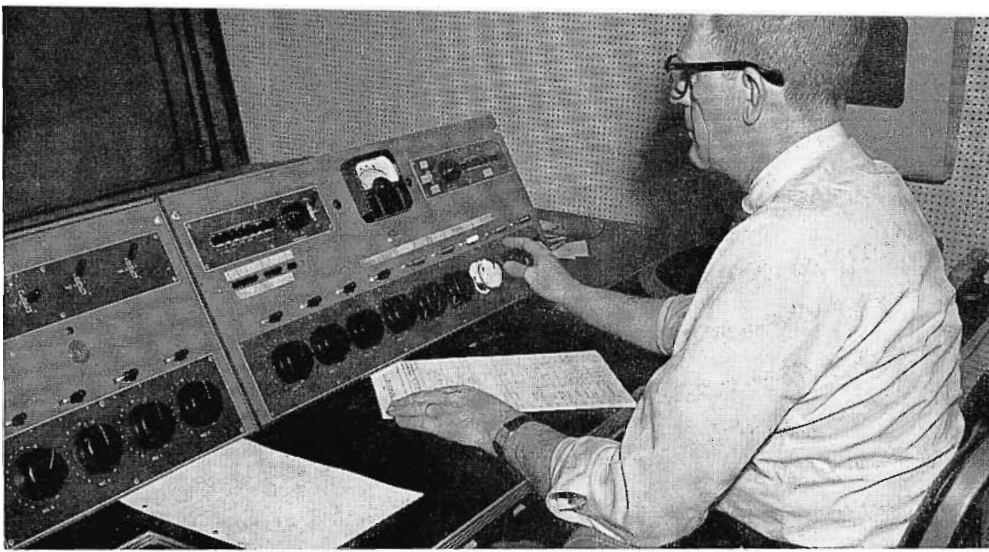
FIG. 20. Remote control video buttons installed on BC-2B audio console permit one-man audio/video switching.
