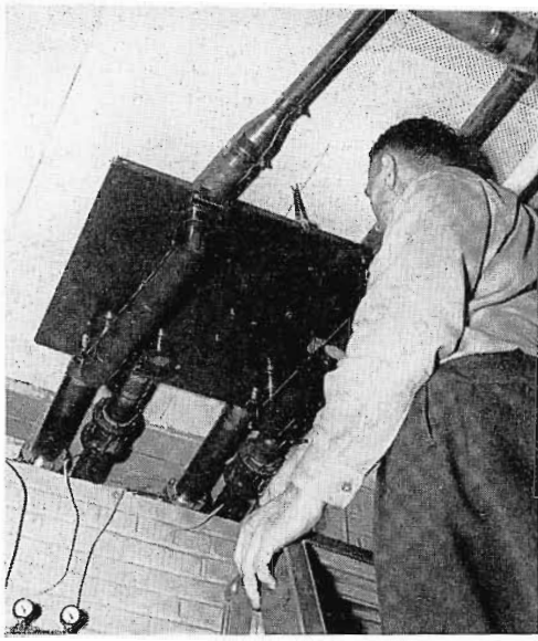
FIG. 27. Ceiling-mounted coaxial switches select R-F feed to either the main 12-bay or the single-bay emergency antennas.
